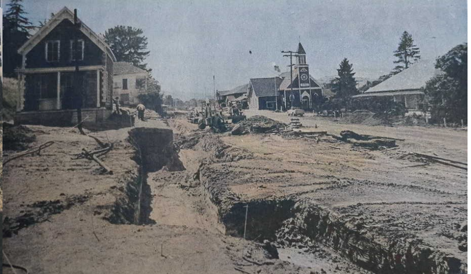
This will be the first view of Novato for motorists taking the DeLong Avenue off-ramp from the new freeway when it opens in late September. The deep channel slicing by the old postmaster's house at left is the excavation for the footing for a concrete block retaining wall which will be faced with Boston ivy.
